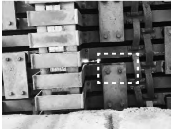
Figure 3. The waterstop is broken.
