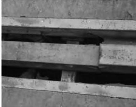
Figure 1. Beam fracture in the expansion joint.
